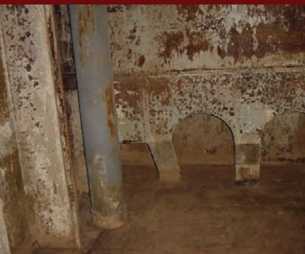
Typical condition of Ballast Tank Coating after a number of years.
