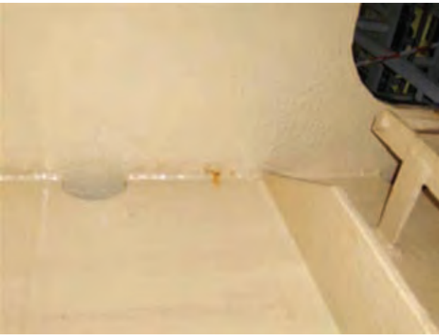
Soltaire, Ballast water tank coating after eight years service.
